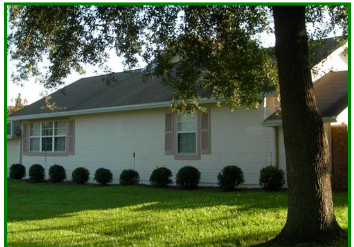
Figure 2: Shrubs along wall are over-trimmed
