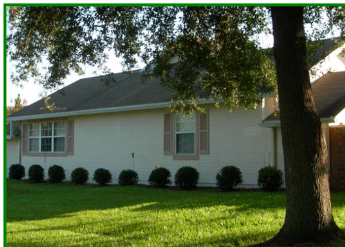
Figure 2: Shrubs along wall are over-trimmed
